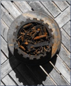
03. BULLETS, TRANSMISSION, AND RUSTED NAILS PULLED FROM A 3/4" OAK FLOOR.
